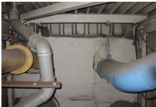
Wall with trowelled loose asbestos
