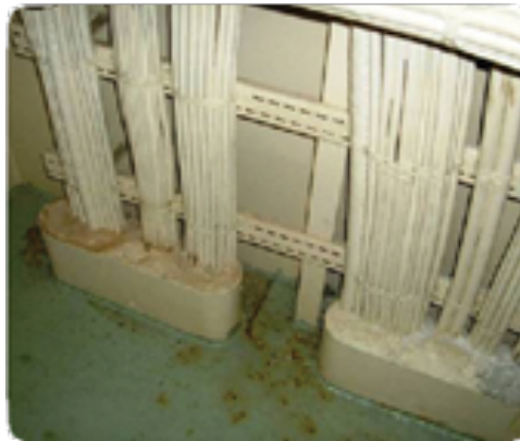
Figure 4. Asbestos-containing cable penetrations used in ships.
