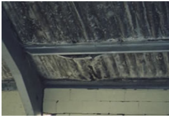
Damaged asbestos cement roof
