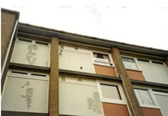
Damaged asbestos paneling
