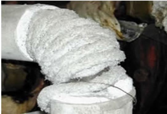
Pipe insulated using both asbestos lagging and rope
