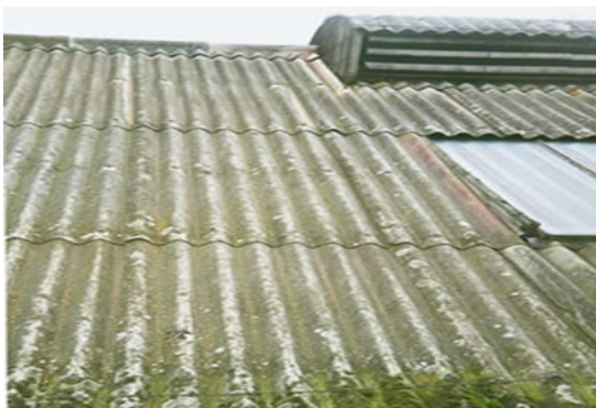
Asbestos cement roof (weathered exterior)
