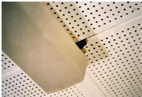
Perforated AIB ceiling tiles damaged around the light fitting
