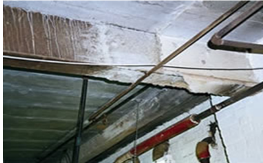
Sprayed 'limpet' asbestos coating which has been partly removed
