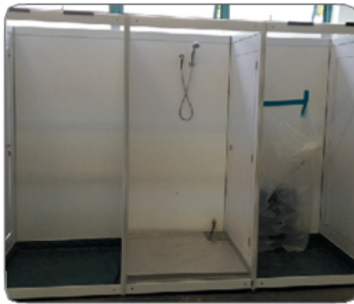
Figure 13. A decontamination facility consisting of 3 separate compartments (clean, shower and dirty areas).
