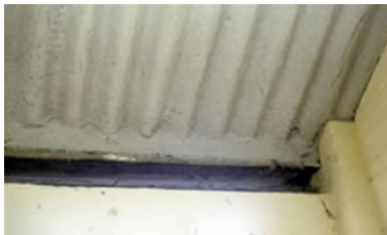
Sprayed 'limpet' asbestos on the underside of an asbestos cement roof
