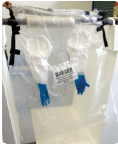
Figure 15: Glove bag containing asbestos waste.
