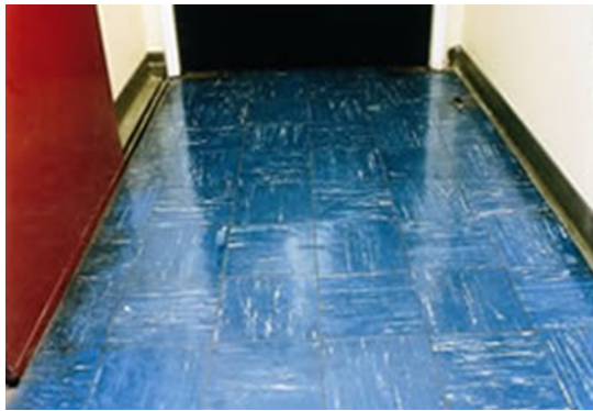
Asbestos-containing vinyl floor tiles
