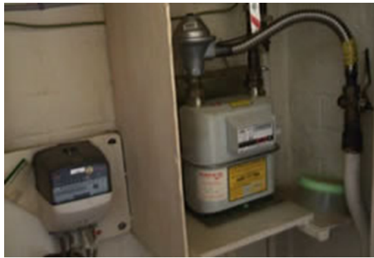
Asbestos paneling around gas meter
