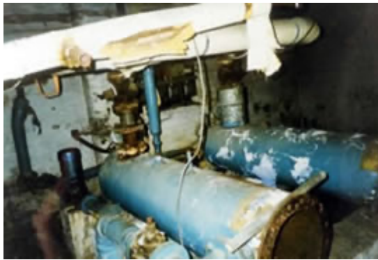
Damaged asbestos pipe lagging and debris
