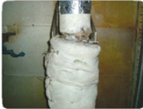
Figure 3. Asbestos cloth wrapping with asbestos lagging of exhaust pipe.
