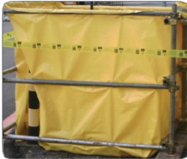
Figure 9. Example of a self-supporting temporary enclosure
