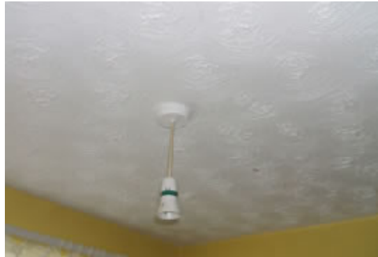
Asbestos texture coating
