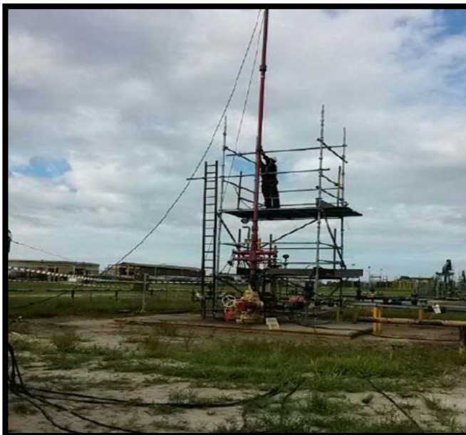
Figure 1 (b) - Static Tower Scaffold for General Purpose
