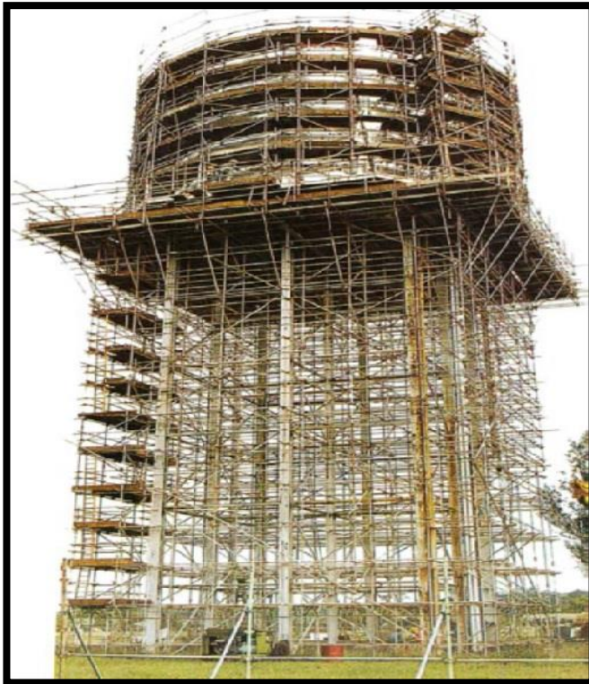
Figure 8 – Combination of Bird Cage, Cantilever and Circular Scaffolding using Tubes and Clamps
