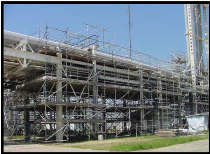
Figure 3 (a) – Independent Scaffold using Tubes and Clamps for Piping and Structure Construction
