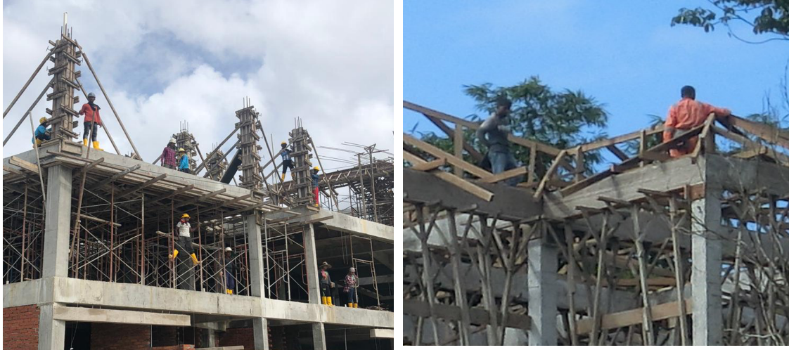
Fig. 1 SHENA Inspection photographs showing Work at Height without proper PPE and controls.
