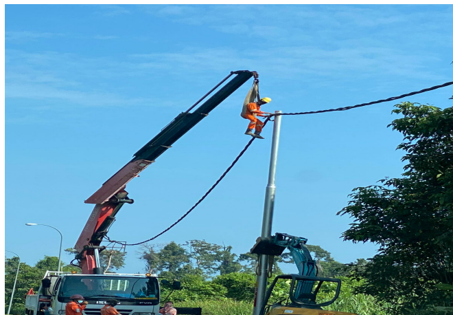
Fig. 1 Photograph received by SHENA showing dangerous occurrence of a man being suspended at height using sling attached to a Hiab Crane.
