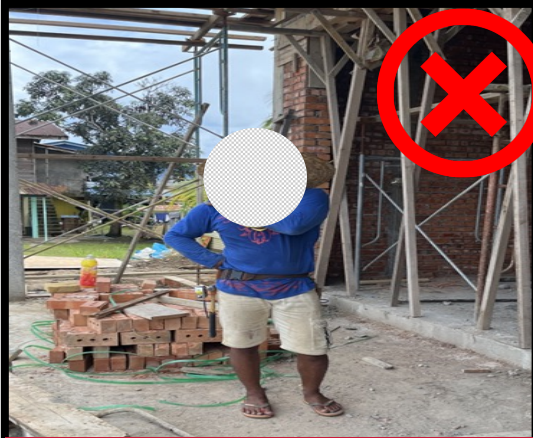
No PPE worn
