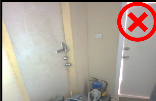
Blocked emergency exit door
