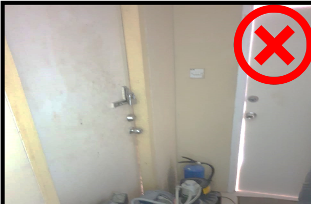
Blocked emergency exit door
