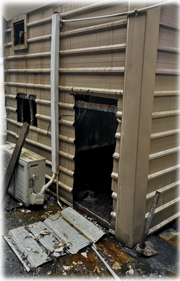
FIRE – CHEMICAL STORAGE / FAULTY EXHAUST FAN
